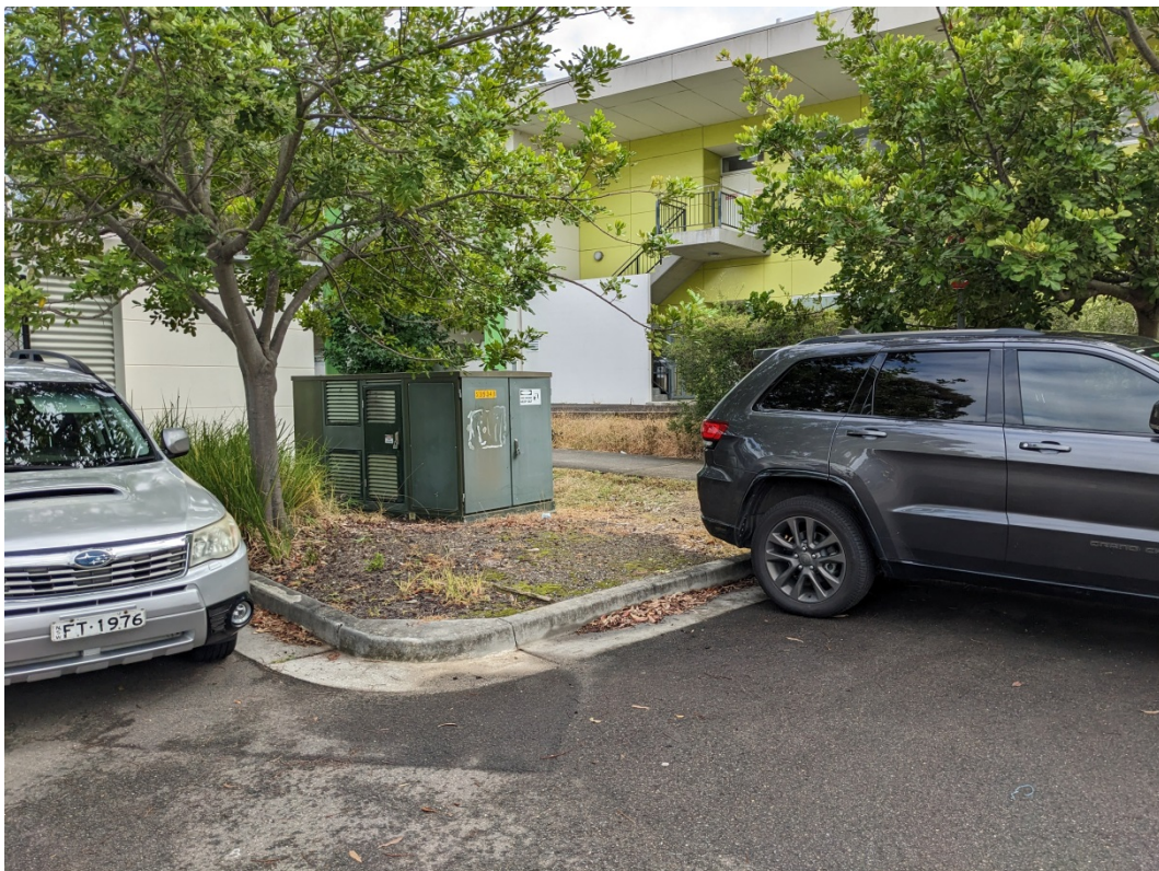
Photograph 6: view of the electricity substation
